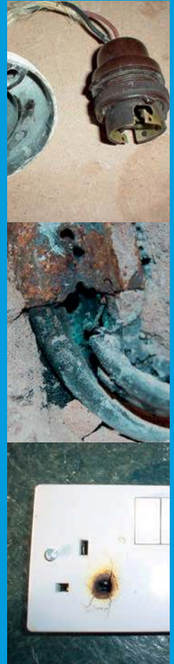
Typical examples of potentially dangerous electrical installations
